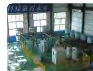
Owning MV full load testing center
