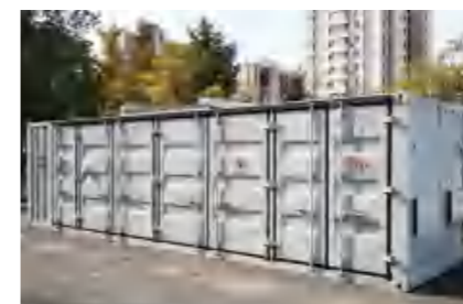
Supplied 45Mvar/35kV SVG with active power filter to Russia Tominsky GOK
