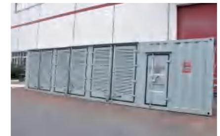
Supplied 20Mvar/33kV SVG to Malaysia 50MW photovoltaic plant
