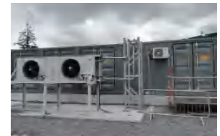
Supplied 8Mvar/10kV SVG to Beinneun wind farm reactive power compensation project
