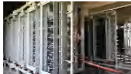
Fig. 3 SVG on-site photos (Indoor power cabinet)
