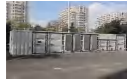
Supplied 14Mvar/33kV SVG to South Korea ASO TAKAMORI Photovoltaic
