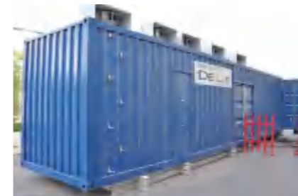
Supplied 10Mvar/10kV SVG to Papua New Guinea national grid
