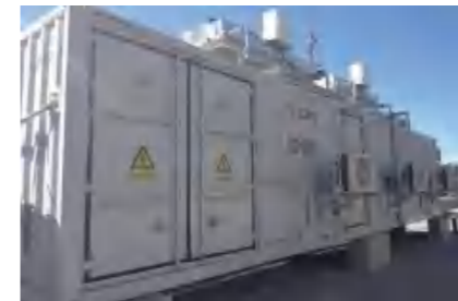
Supplied 40Mvar/34.5kV SVG to Mexico Diram-deacero electric arc furnace (with 40 Mvar FC 2sets)
