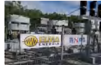
Supplied 100Mvar/31.5kV SVG to Poland ELMA company CMC steel mill electric arc furnace(with FC)
