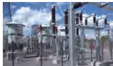
Fig. 2 SVG on-site photos (outdoor primary equipment)
