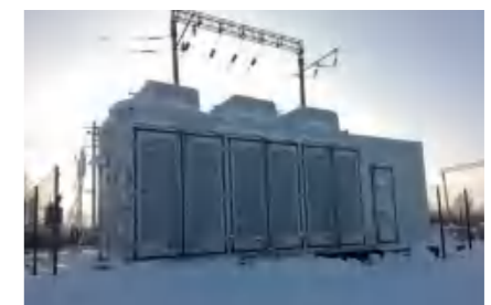
Supplied 10Mvar/27.5kV SVG to Russian electrified railway (-30 C working temperature)
